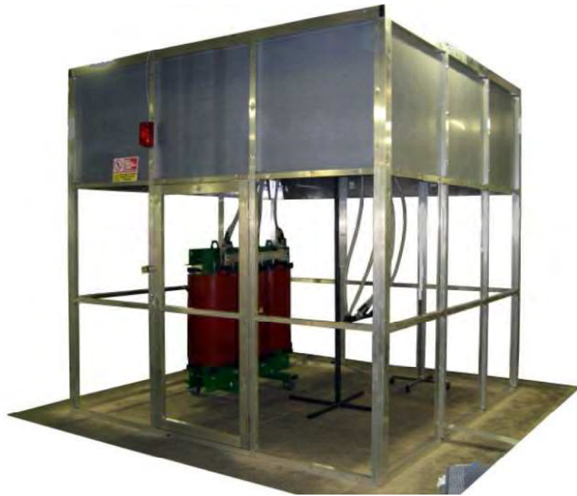
Figure 115 Shielding on the substation ceiling and on the side for 1m high (Conf. 2)
