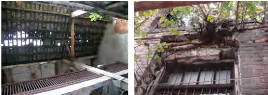
Figure 86 Details of Former Residence of Cheng Qian Before Restoration
