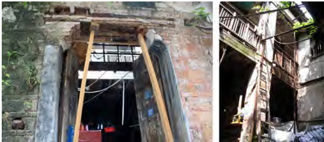
Figure 92 No. 26, Fengjiawan Lane in Need of Restoration
