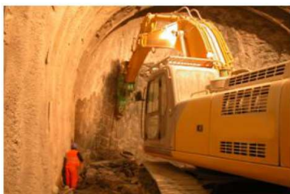
Fig. 4. High Hydraulic Energy Hammer at work while a second worker provides the machine operator with visual help and “tries” to reduce the airborne dust pollution by spraying water onto the face
