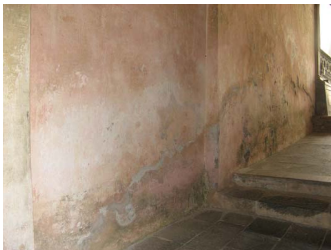
Figure 3. Detachment of historical plasters because of the rising damp effects due to capillary action at Sacro Monte di Varallo
