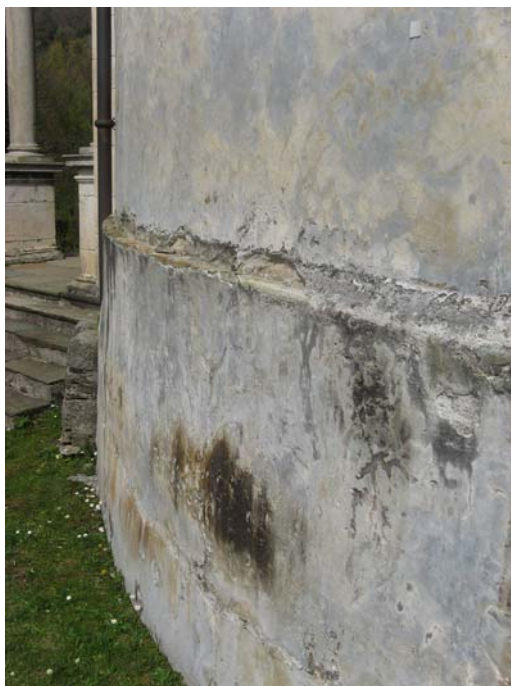
Figure 2. Detachment of historical exterior plasters at Transfiguration Chapel because of the rising damp effects due to capillary action or rain infiltration
