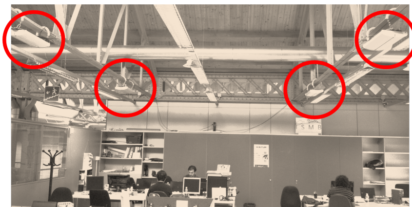
Figure 4.4: The antennas of RFID reader on the ceiling.
