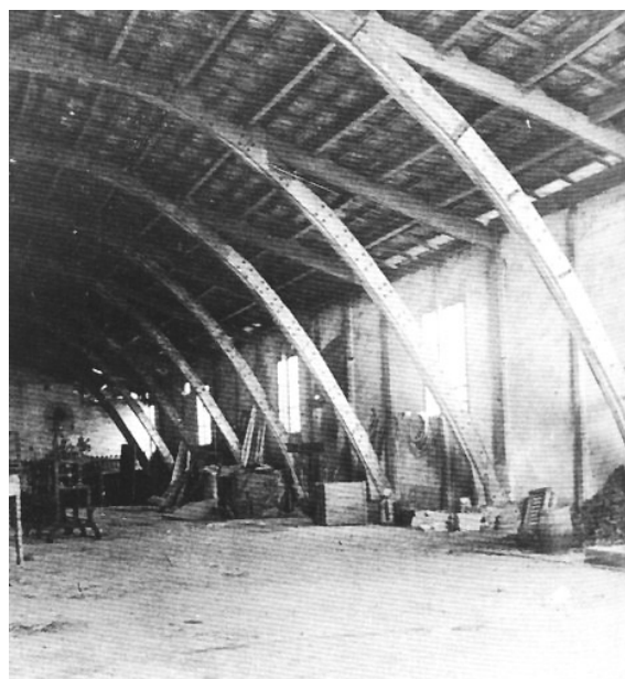
Figure 10 – The Pavilion of the Societat Obrera Mataronense, Matarò, Spain. The wooden arch structure.
