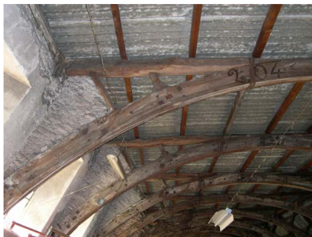
Figure 8 – The former Gallo wool mill, Sagliano Micca (Biella). Detail of the assembly system of the boards. (photo Mattone).
