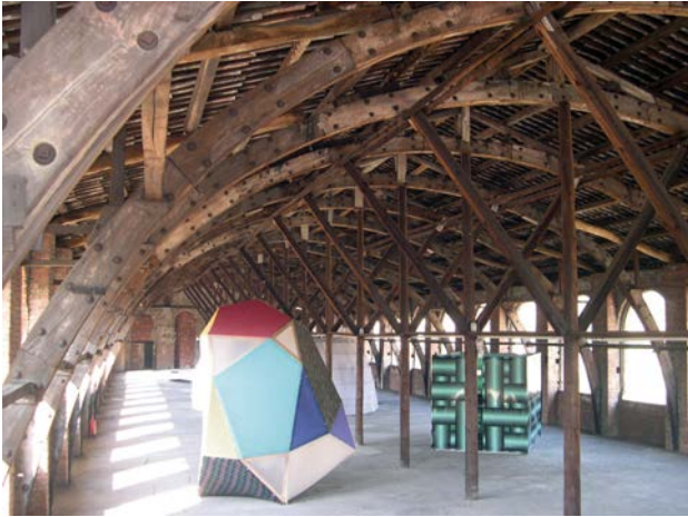
Figure 4 – The former Trombetta wool mill, Biella. The wooden arch structure. (photo Mattone).
