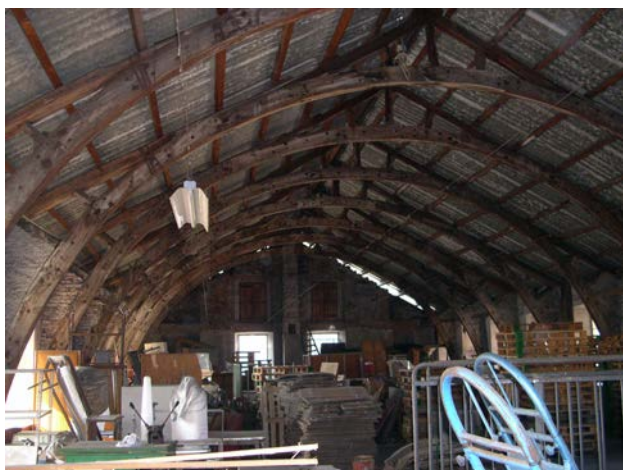
Figure 7 – The former Gallo wool mill, Sagliano Micca (Biella). The wooden arch structure. (photo Mattone).
