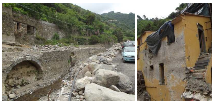
Figure 3: Examples of damages to buildings along the Vernazzola stream.
