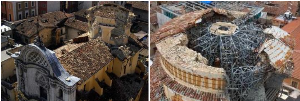
Figure 4.8 - Church of Anime Sante in L'Aquila after the 2009 earthquake (left) and the temporary scaffold (right).
