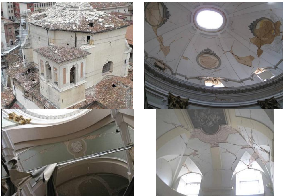
Figure 4.36 - Damage due to the 2009 earthquake: (a) Lantern completely destroyed, the damage on the tiburio and on the bell tower, (b) Damage on the dome's groins, (c) detachment between the main body and the dome, (d) Vault of the sacristy.
