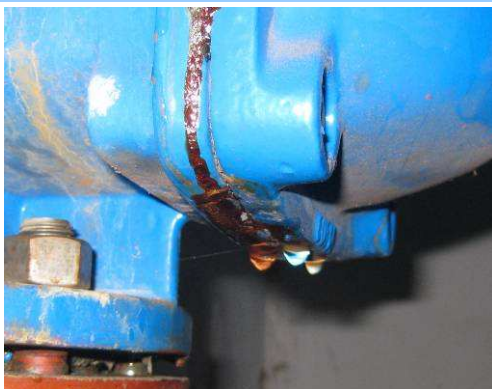
Water leaks pictures
