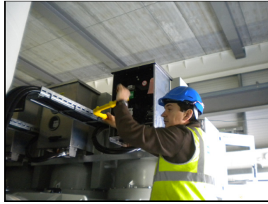
Figure 23: Operator trying to reach while standing on a ladder the manual gear to open the switch in case of failure of the automatic system for the side bay.
