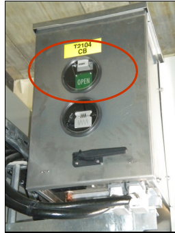
Figure 21: Position of the indicator (above 2mt. high and difficult to read in between bays)
