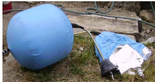
Fig. 2 Blocking balloons with frustum of cone plugs to stop the pipe holes; the deflated balloon is strengthened by an aluminium sheet which constitutes a protection against sparks originated by welding operations.
