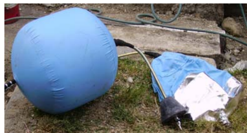
Fig. 2 Blocking balloons with frustum of cone plugs to stop the pipe holes; the deflated balloon is strengthened by an aluminium sheet which constitutes a protection against sparks originated by welding operations.
