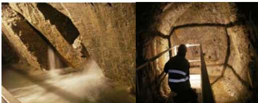
Fig. 6: On the left: Water flows from the fractured mass giving rise to the Sorgente di Tenda; on the right: Excavation face of the tapping tunnel
