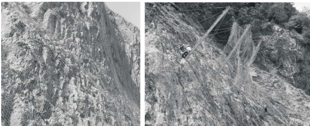
Fig. 6. Details of the drapery wire meshes and net fences installed on the rock slopes to protect the quarry yard
