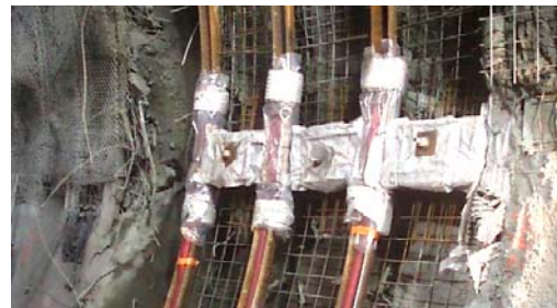
Figure 3. Highly Deformable Concrete (HiDCon) elements during installation between the TH steel ribs and before shotcrete placement.
