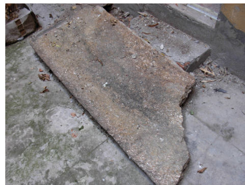
Figure 2: The broken balcony slab of figure 1.
