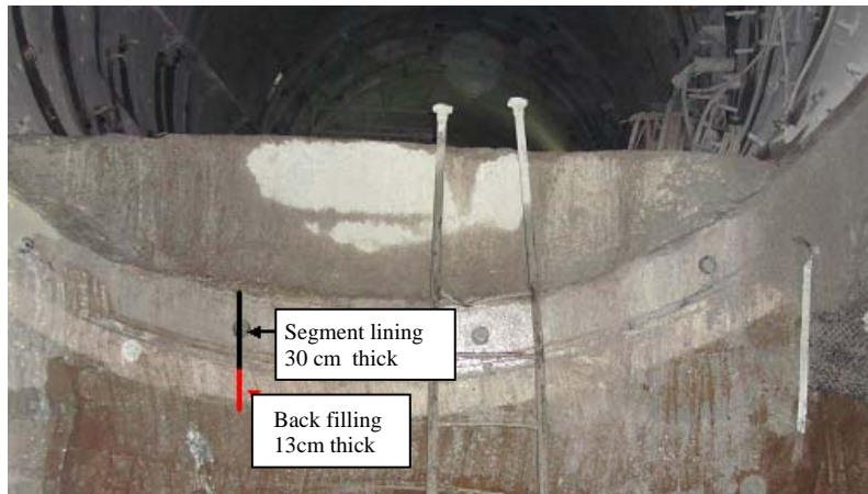
Figure 2 – Example of backfilling in a metro tunnel in Italy (Prof. Pelizza’s pictures archive)
