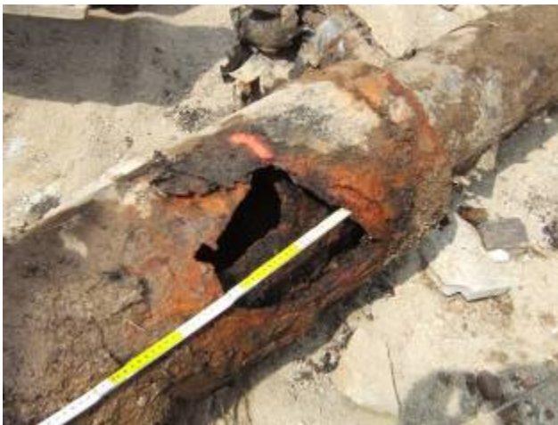
Fig. 6 – Gas pipe damage “A”
