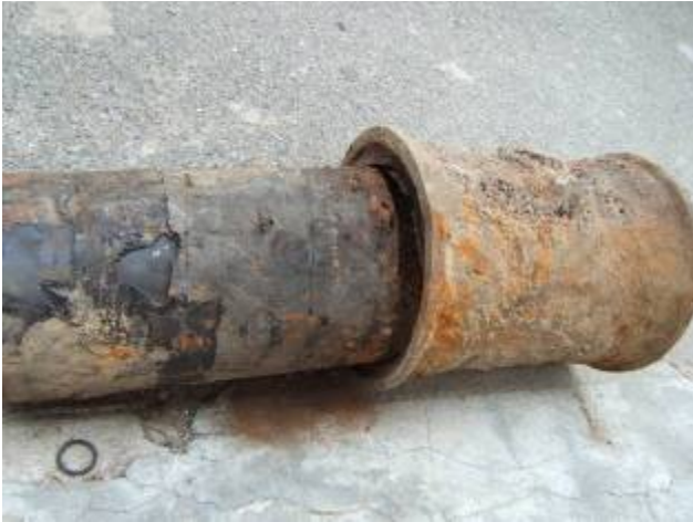
Fig. 4 – Gas pipe damage “B”
