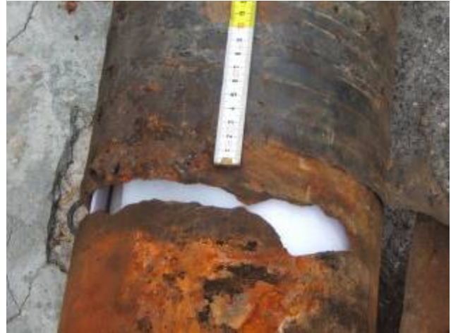
Fig. 5 – Gas pipe damage “B”
