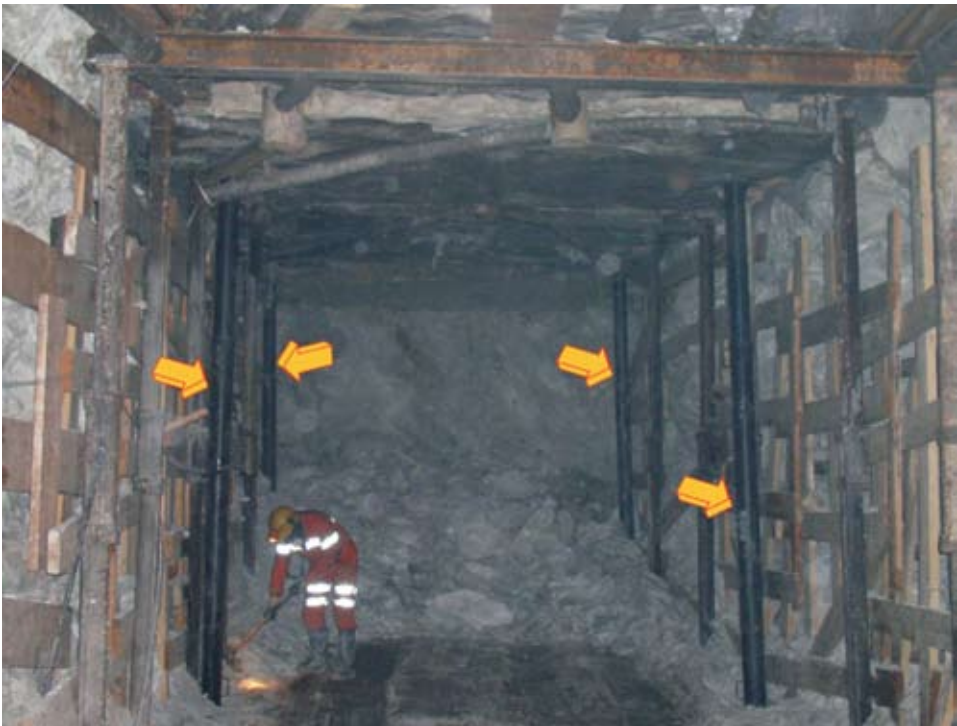
Figure 1. View of a drift supported by timber sets and hydraulic (arrows) and mechanical props
