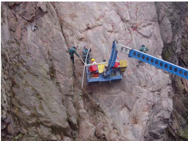
Fig. 11. Charging phase using a mobile platform. The charges were pre-prepared inside a PVC pipe to facilitate ease of placement into the drill holes.
