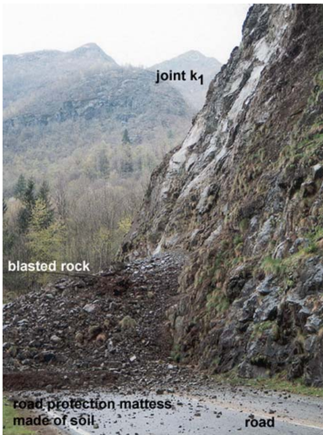
Fig. 6. Result of the blast. It is possible to see the joint k_1 that was behind volume n. 1 and the good fragmentation of the blasted rock.
