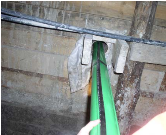
Figure 12. Detail of the installation of the asymmetric casing along a transversal drift in the Rodoretto mine for a length of 26m
