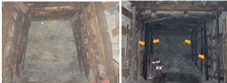
Figure 1. View of a drift supported by timber sets and hydraulic (arrows) and mechanical props
