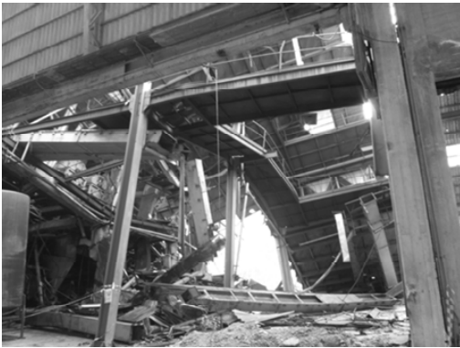
Figure 5. Partial collapse of the steel/reinforced concrete structures sustaining Building “A”.
