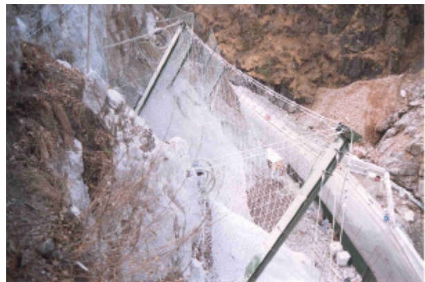
Figure 1. View from the upper part of the rock slope: some net fences are visible and in the right side the existing road.
