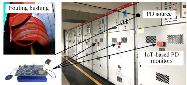
Fig. 13. Online PD monitoring of MV switchgears via IoT-based PD monitors.
