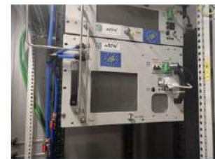
Figure 2 Installed electrolyser at ZEM module
