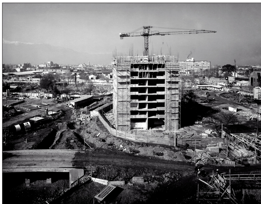
Figure 14: Demolition and construction, simultaneously, of the San Borja Remodeling, c. 1968. Special Archive of Architecture, FADEU Archive of Originals, Pontificia Universidad Católica de Chile. Material compiled and donated by Patricio Gross.
