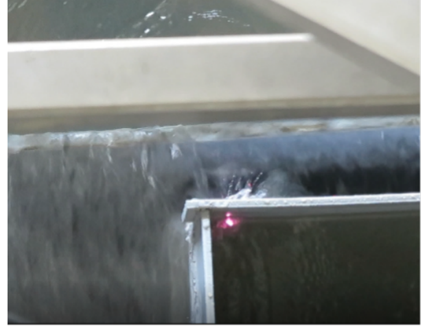
Fig. 5: Electrical sparks between the spilling water and the tank of another phase.
