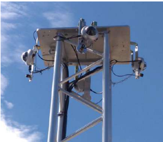
Fig. 2 – Weather station installed at NOI TechPark in Bolzano
