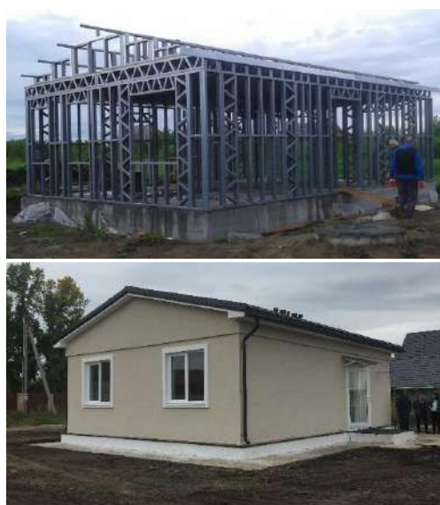
Fig. 1 – The building during (a) and at the end of the construction phase (b). Picture by Giovanni Manzini, 2019
