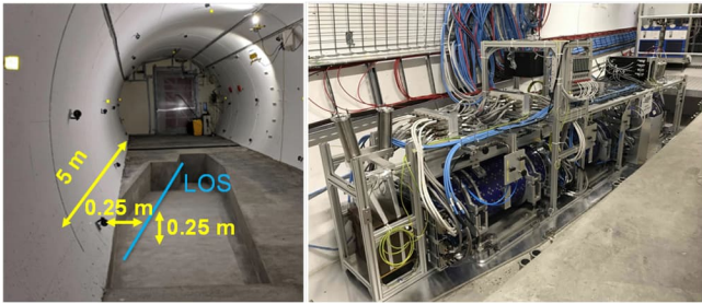
Fig. 3. TI12 tunnel before (left) and after (right) FASER installation.
