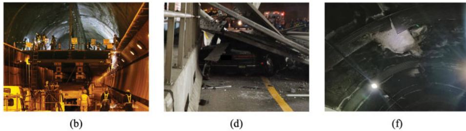
Figure 2. Tunnel local collapses that drove the development of modern tunnel guidelines: (a) Sasago tunnel ceiling panel fall and (b) subsequent refurbishment 16,20 ; (c) Ted Williams tunnel ceiling panel fall and (d) vehicle with a fatally injured occupant beneath 22 ; (e) Berté tunnel concrete vault collapse and (f) resulting cavity in the lining 23
