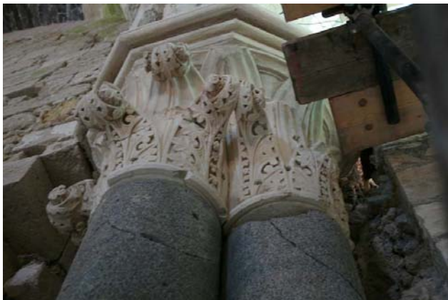
Figure 12 Cracks in the marble shafts of the trilobate columns deriving from the stress concentration due to eccentric axial loads.
