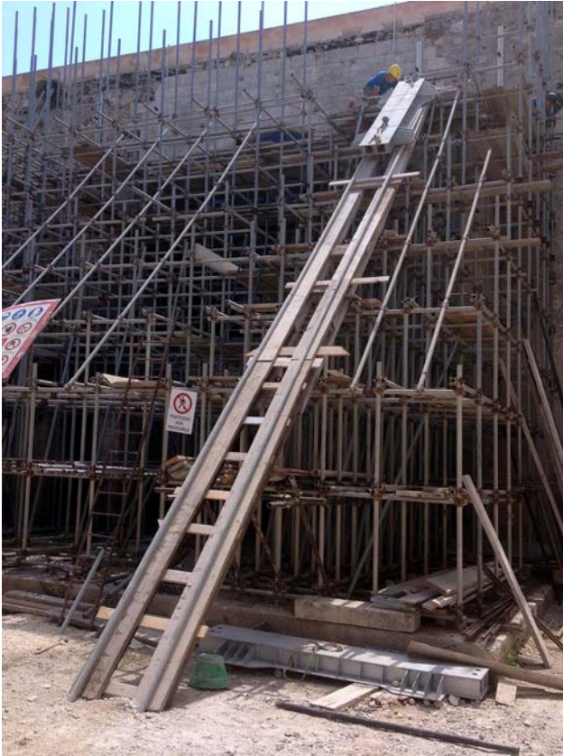
Figure 28 The inclined plane fixed to the existing scaffolding employed to pull up the stiffened plate.
