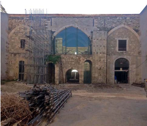
Figure 30 The façade during scaffolding dismantling; only a portion is still present on the back of a buttress.
