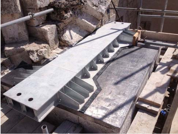
Figure 27 Picture of the stiffened top plate over the buttress, levelled by mortar and a copper coating
