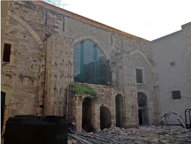
Figure 31 The removal of the scaffolding is complete and its concrete foundation almost demolished.
