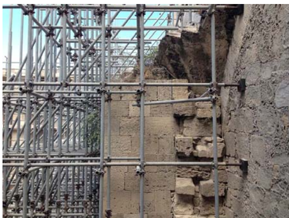
Figure 8 A lateral view of the stonework arrangement of the right buttress. From the top of the buttresses, the surviving tas-de-charge portions of the vaults, which collapsed or were demolished in the 18 th century, can be seen.
