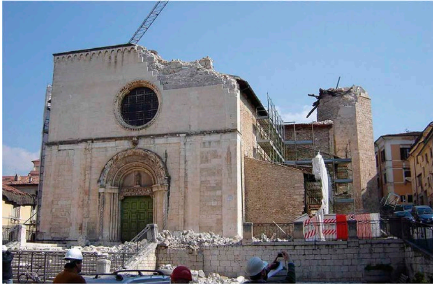
Fig. 12. Damage due to the earthquake of 6 April 2009. The right corner of the façade has collapsed, as also the top of the bell tower, which, falling, also badly damaged the roof of the transept. The collapse shows that the stone cladding consists of thin stone slabs stuck onto the wall; moreover, the first row of stone cladding, which remained in place, does not seem to extend beyond the part (trapezoidal pilasters) where Moretti reused the stones elements of the previous façade for his restoration (top and lower left). Inside the church, the cracks follow the lines of the Baroque façade (lower right).
