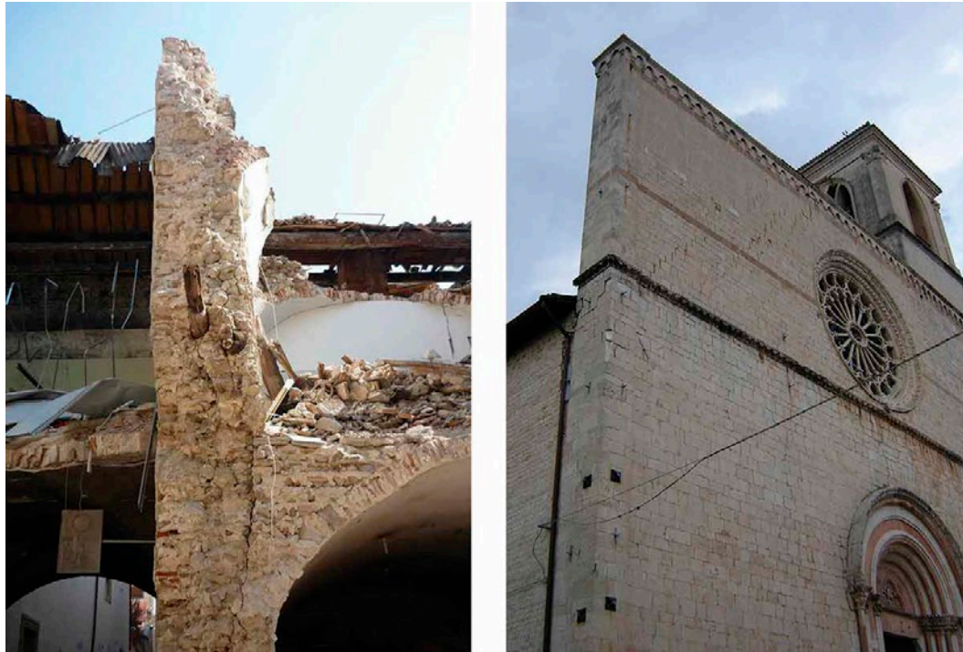
Fig. 1. L'Aquila: wooden log ( radiciamento ) in a shear wall (on the left). L'Aquila: the effectiveness of wooden logs inserted in the façade of the church of S. Silvestro preventing its global overturning (on the right).
