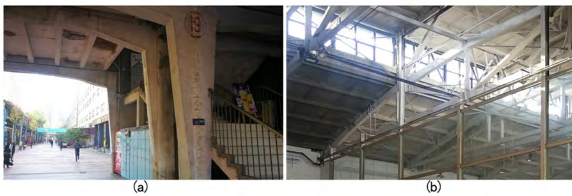
Figure 27. The Chengdu Hongguang Electronic Transistor Factory: (a) the reinforced concrete structure of Assembly Workshop (b) the steel frame roof truss of Testing Workshop.
