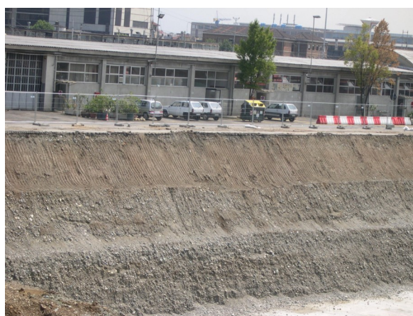
Fig. 17 - An approximately 15 m deep recent building excavation within Turin (Giordano Bruno Street, G in Fig. 14) shows the sequence formed by gravelly and sandy outwash sediments, supplied by the Dora Riparia River during the Upper Pleistocene.
