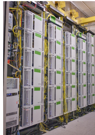
Figure 3.10: A photo of the network equipment.
