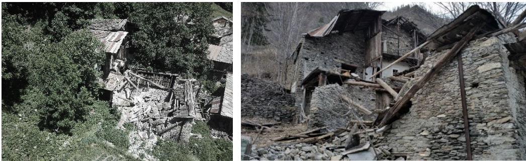
Figure 85. Damaged building of the hamlet of Pomieri (photo by drones).
