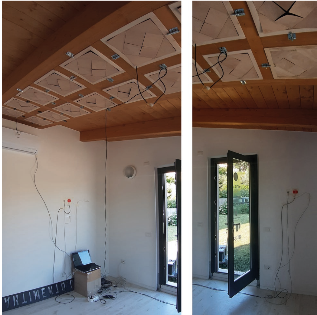
Fig. 2. Thermocouples, fluxmeters, temperature and humidity probes and anemometers inside the test room.
