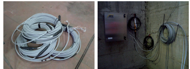
Fig. 5 - Water temperature measuring chain (PT1004/Pt) installed in S2-control piezometer of the Politecnico of Torino open-loop GWHPs
