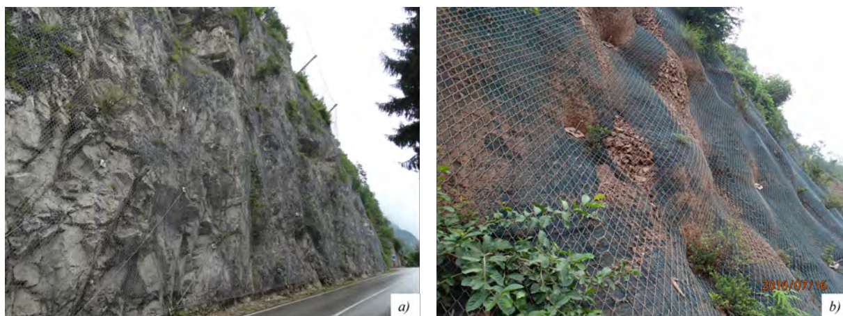
Figure 1. Reinforced drapery meshes with (a) retaining ropes, i.e., secured drapery, and with (b) spike plates, i.e., pinned drapery.
