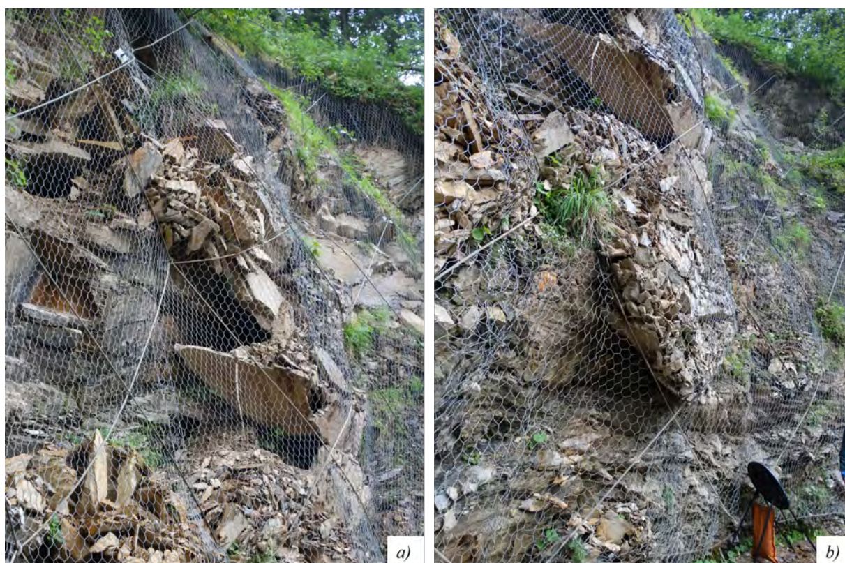
Figure 2. Beneficial effect of the ropes, which prevent failure diffusion near the anchors (a) and provide constraints for the mesh similar to those of standardized laboratory tests of UNI 11437 (b).
