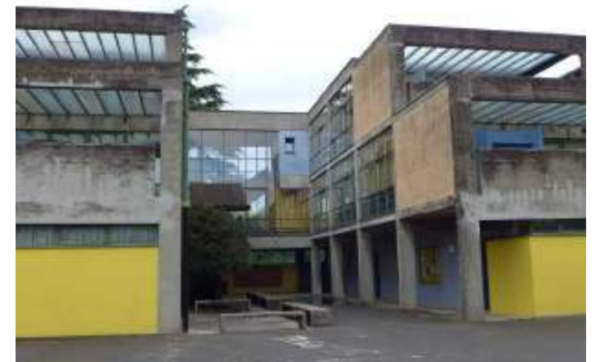
Fig. 2. Flora Ruchat-Roncati, Aurelio Galfetti and Ivo Trümpy, School in Riva San Vitale , 1962–4, 1970, Photographer Katrin Albrecht, 2017. Courtesy of Katrin Albrecht.
