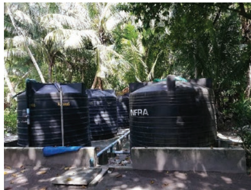
Figure 2. Public water tank used by the inhabitants of Magoodhoo to collect rainfall water for daily use.
