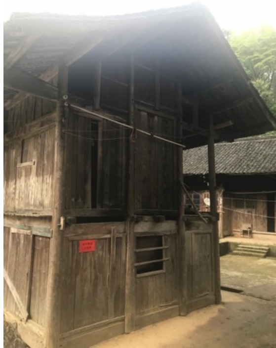
Figure 117: the dilapidated dwelling with the Red Sign Showing the Dweller Has New Houses in the village. Source: author's photo.
