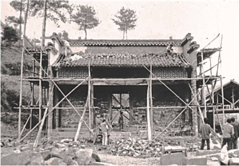
Figure 6: Demolished and reconstructed portal of the Qiankou dwellings Source: Report of MQR.
