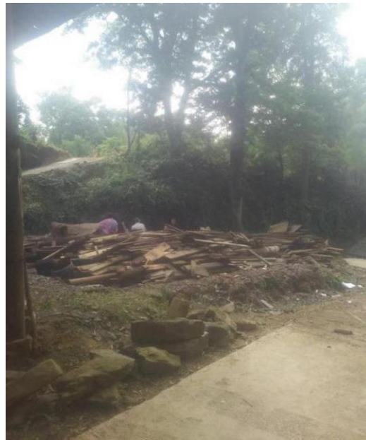
Figure 120 The demolished wooden dwelling. Source: Photo taken in 2018 by the village head Wu Jiayong.
