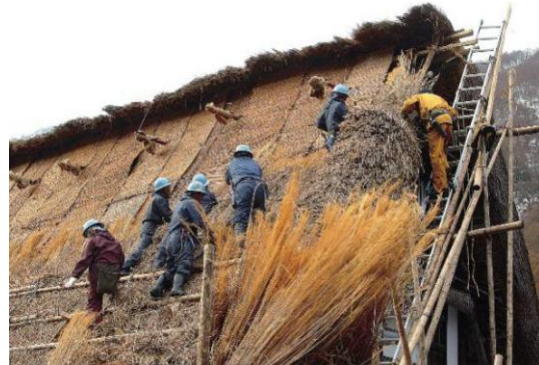
Figure 133: Villagers of the Preservation Organization working on the straw-thatch roof Source: Ahmad, Radzuan & Fukami, 2013
