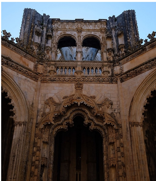
Fig. 1 Facade and ornaments with orange patina at the Imperfect Chapels, Batalha Monastery
