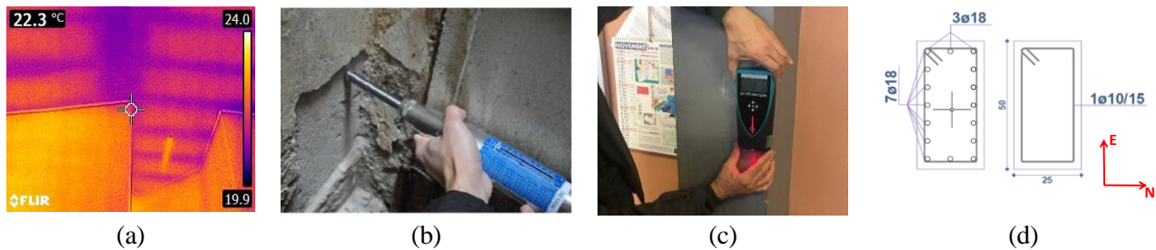
Figure 3. Thermal camera test (a), sclerometer test (b), pachometer test (c), and column cross section (d)
