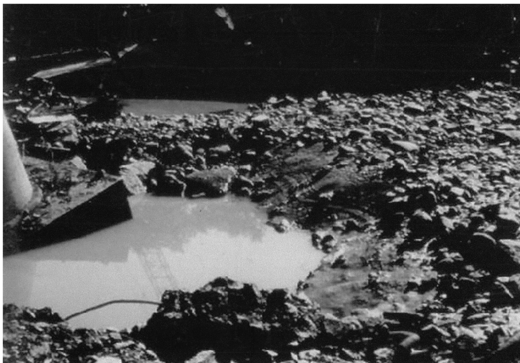
Figure 3.2: Pier local scour holes at Schoharie Creek Bridge (from Lagasse and Richardson, 2001).
