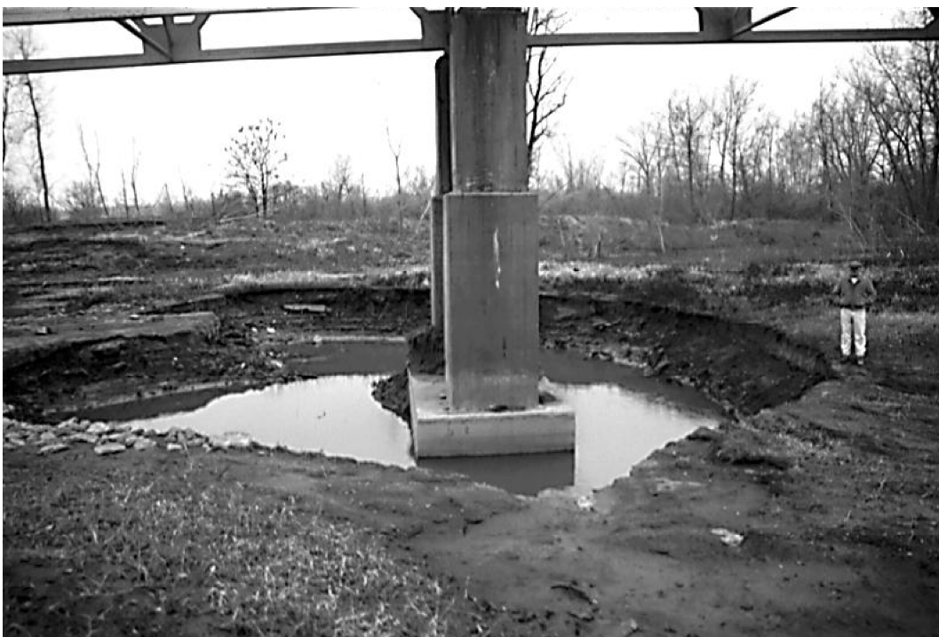
Figure 2.2: Effects of local scour around a bridge pier (from Sheppard and Renna, 2005).
