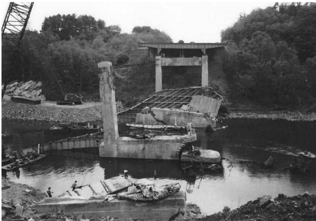
Figure 3.1: Collapse of the Schoharie Creek Bridge (from Delatte, 2008).
