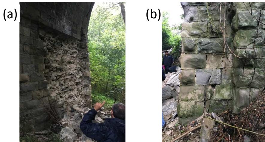
Fig 7 – Roman-era bridge along the Trisungo route (Tufo area – Arquata del Tronto): (a) spalling and (b) cracking of exterior masonry elements. (N42.735389, E13.253611, September 7 2016).
